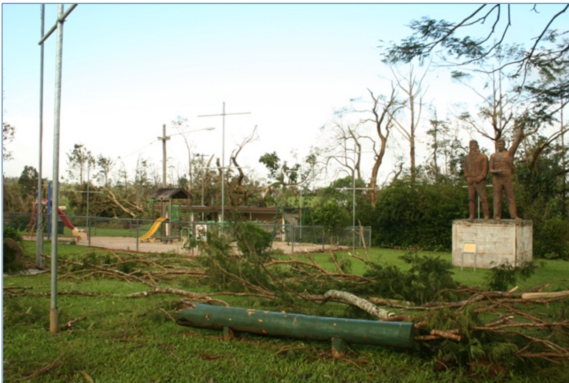
Figure 4 Infrastructure Damage after Cyclone Larry, Mission Beach, 2006 (Source: http://www.rainforest-facts.com/ via Wikimedia Commons)
