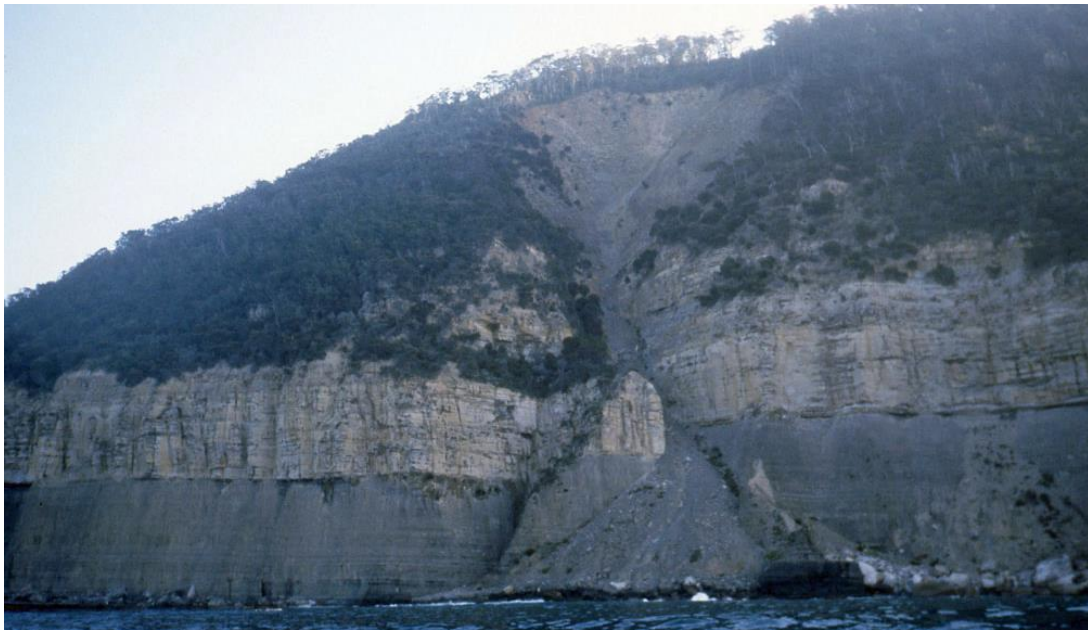
Figure 2: A large active slump in hard Triassic sandstone coastal cliffs at High Yellow Bluff. Although the cliffed hard rock coasts of this compartment are generally stable and resilient, rock falls and slumping do occur sporadically and are likely to become more frequent with ongoing sea-level rise. Photo by C. Sharples (1994).
