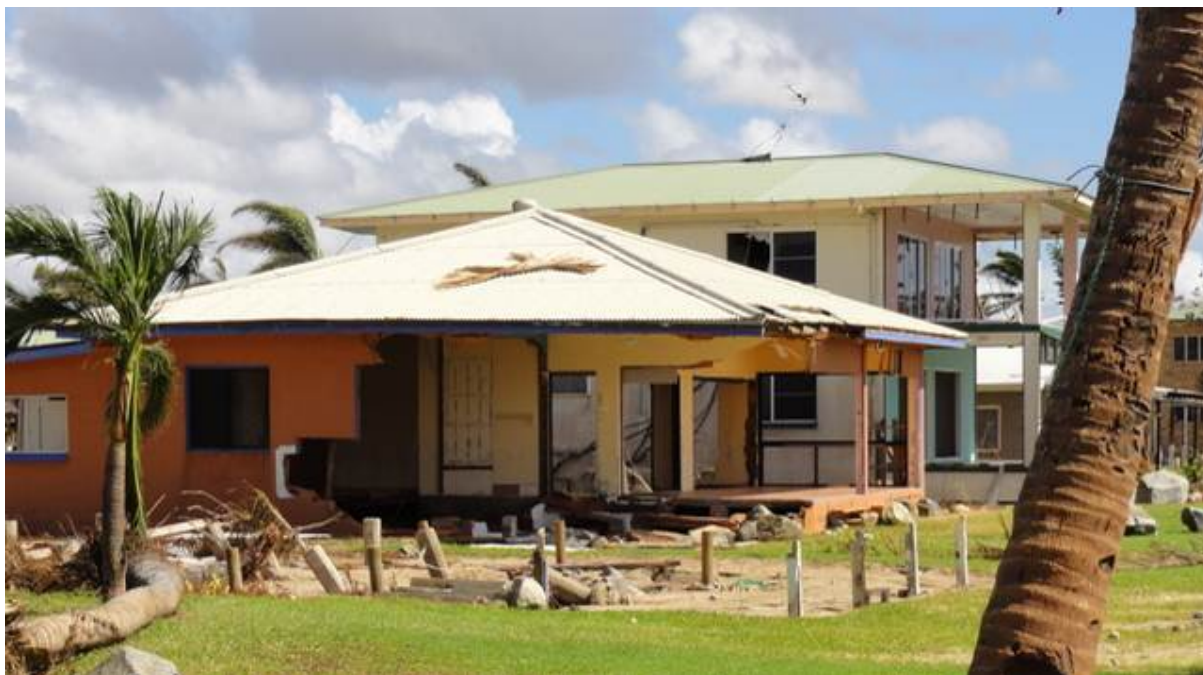
Figure 33: Coastal inundation damage due to storm surge associated with Cyclone Yasi. Note the missing house in the foreground.
