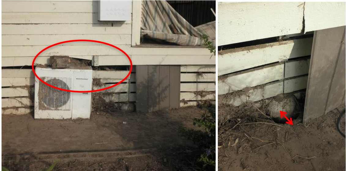
Figure 13: Dynamic debris impact of a fence paling on a home. Right image shows the resulting lateral displacement of a pier foundation.
