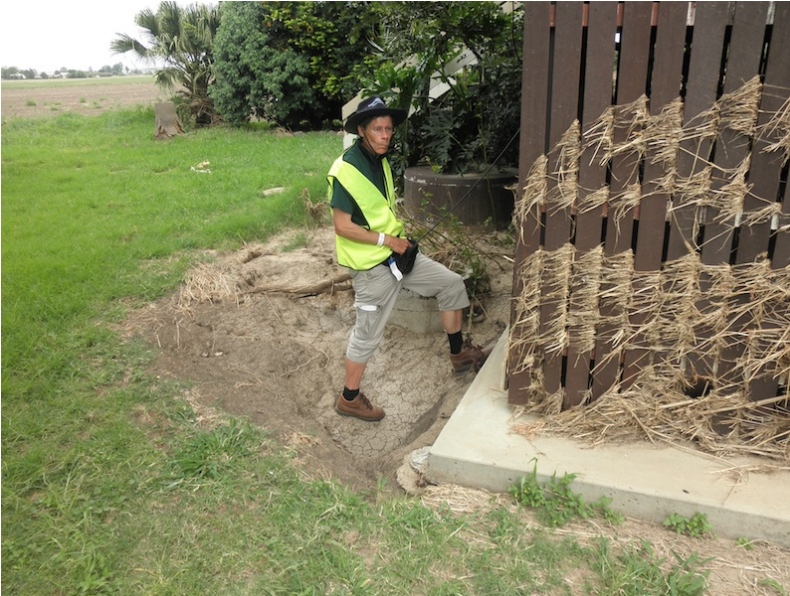
Figure 14: Erosion around corner of foundation. Note the debris caught in the palings suggest a decrease in water depth and therefore an increase in water velocity around the edge of the home.
